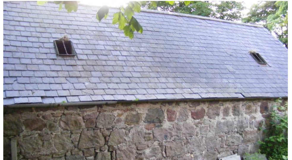
Photo 10: Eastern elevation of Mill building. Roof has several missing slates but is mainly in good condition. Windows are broken allowing water inside contributing to the damp. Ridge appears intact.
