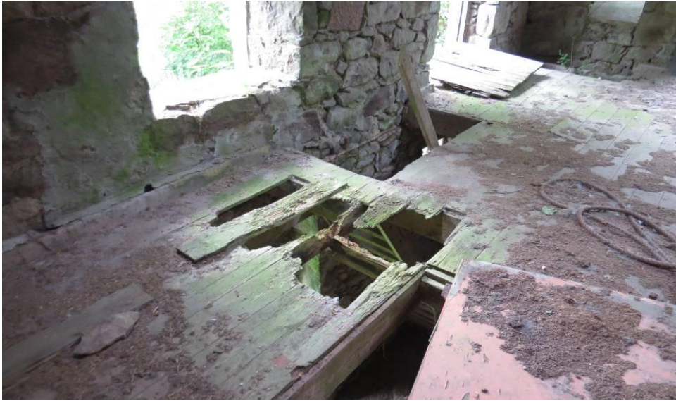
Photo 12: View of staircase from ground floor to lower ground floor. Area is dangerous with rotten floorboards and some joists are not attached to the wall.
