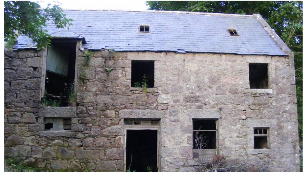
Photo 5: West elevation of mill. Plants are growing from cracks in places show wall is damp. Some loose and missing slates on roof provide limited bat roost potential. No evidence of bats found.
