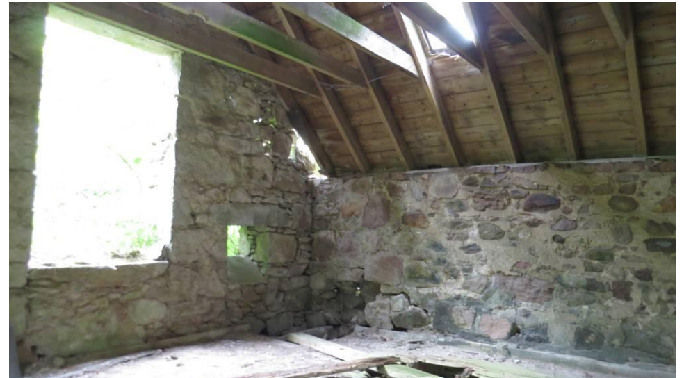
Photo 11: North gable. Large hole in northeast corner of the wall. Roof and floor rotten in places. The building is in poor condition and becoming dangerous.
