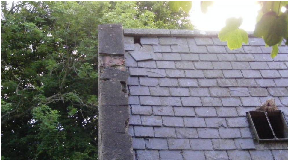
Photo 8: South gable end. A loose slate has caused a small hole in the roof contributing to the dampness inside the mill and in the roof. Lifted and missing slates provide limited roosting potential. No evidence of bats was found.
