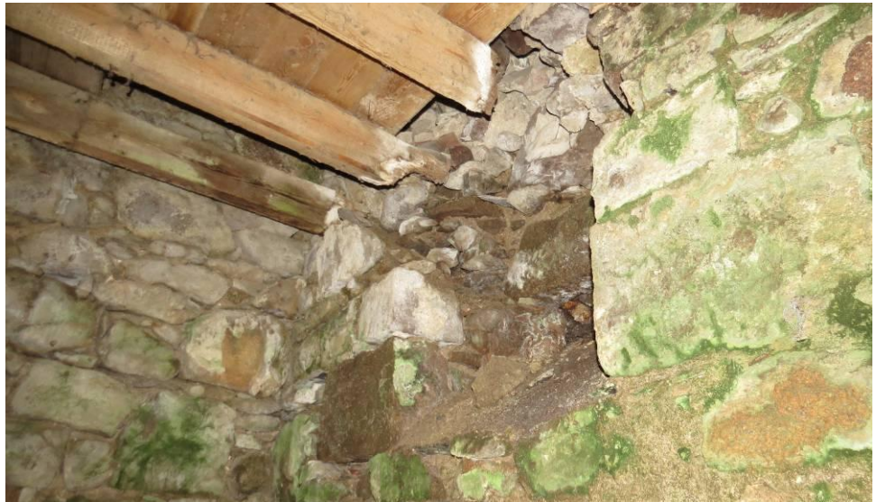
Photo 15: Lower floor ceiling beams rotten and dangerous. The wall is very damp with no bat roost potential.
