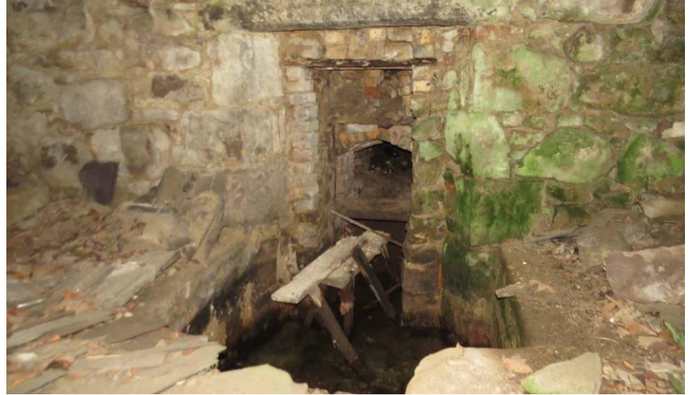
Photo 14: Lower floor, north gable of main building. Grain drying kiln floor has fallen in. The walls are damp and have no cracks. The gain kiln has a collapsed chimney. Inspection showed no evidence of bats
